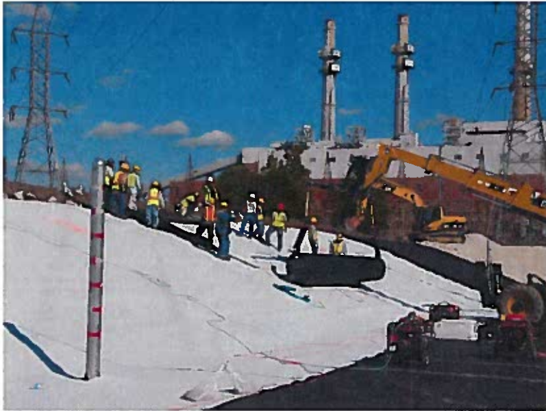
Installation of 16 oz non-woven geotextile and white HDPE liner, looking at northeast corner of South Ash Pond #3.
