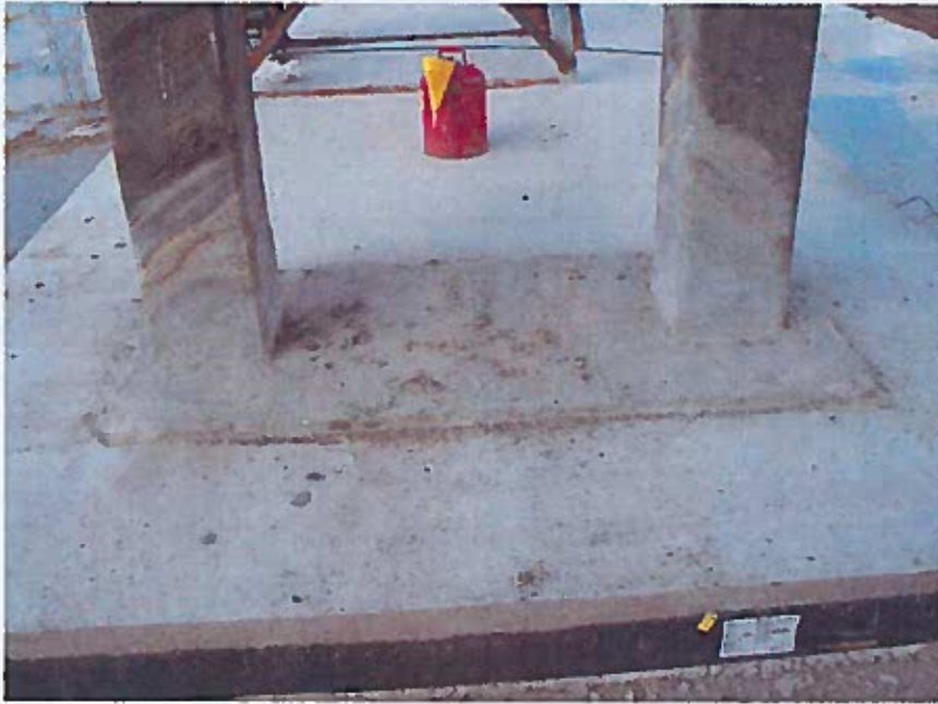
New concrete base with welding strip around influent pipe support posts (looking west).
