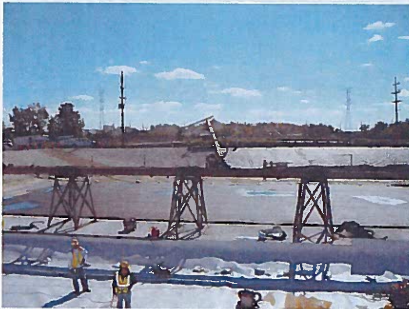
Looking south, placing liner on south slope and crew working on welding toe of slope.
