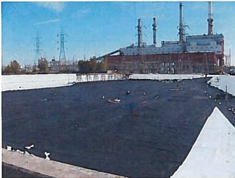
South Ash Pond #3 looking east of the 12oz non-woven geotextile placed above the liner.
