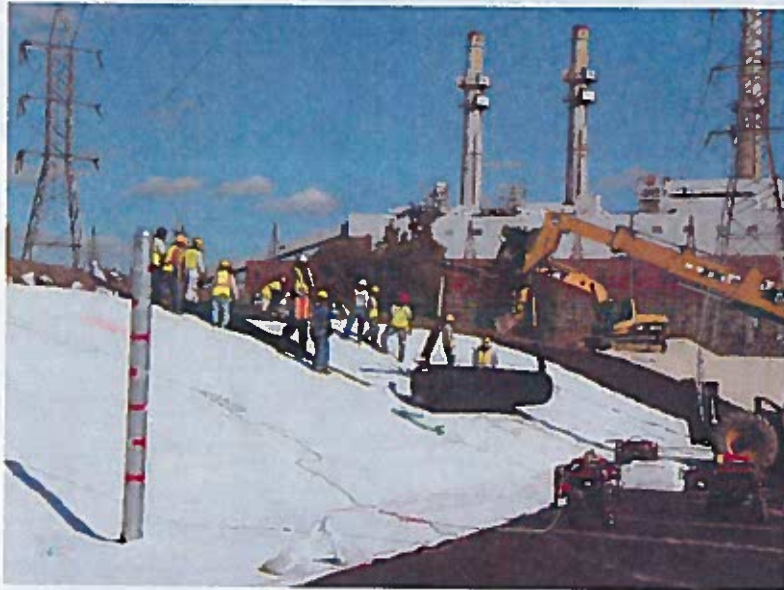
Installation of 16 oz non-woven geotextile and white HDPE liner, looking at northeast corner of South Ash Pond #3.
