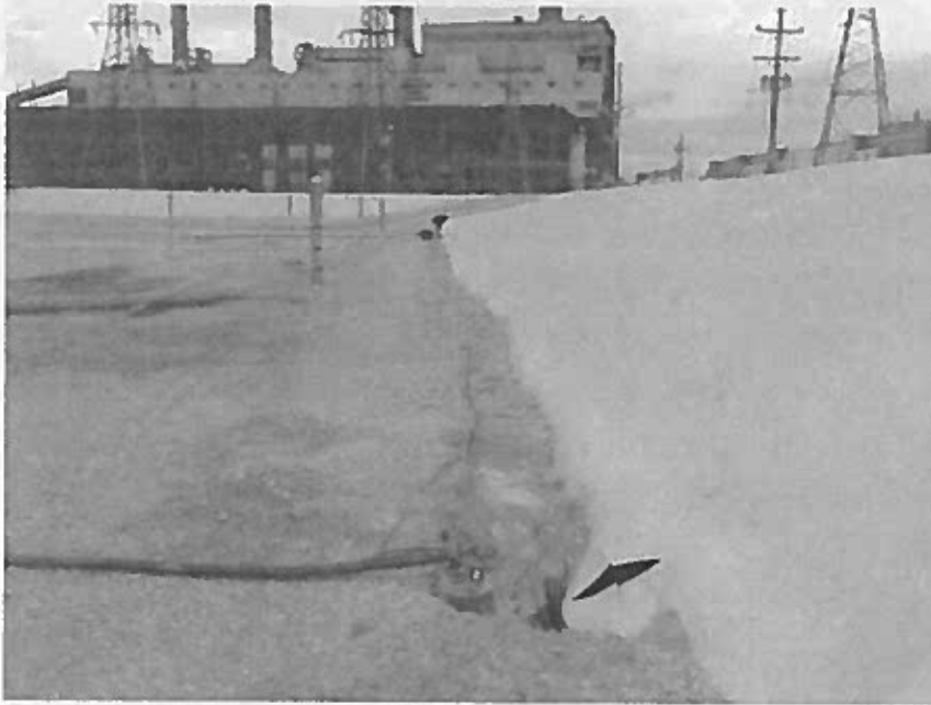
Hole in liner for water removal on south toe of basin (looking east).
