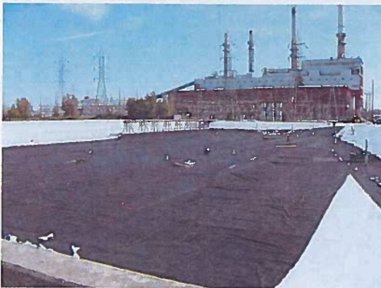
South Ash Pond #3 looking east of the 12oz non-woven geotextile placed above the liner.
