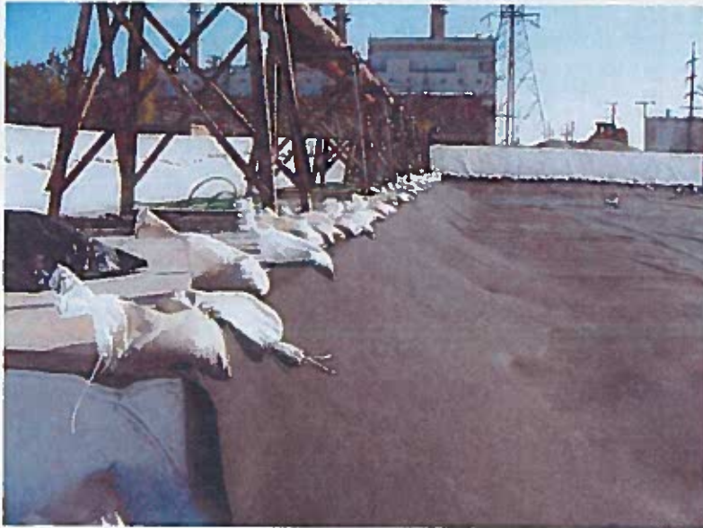
Liner connected to weld strip along concrete pad, and 12oz non-woven geotextile placed above the HDPE liner to protect the connection and liner.
