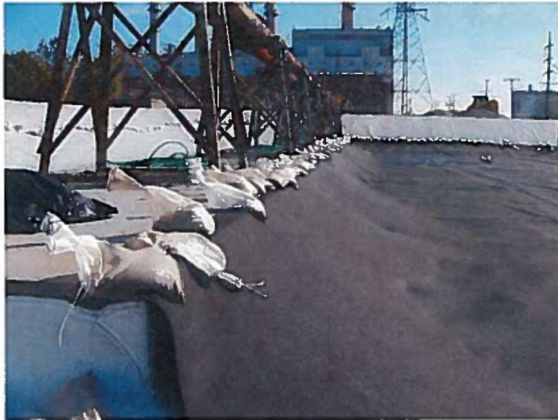
Liner connected to weld strip along concrete pad, and 12oz non-woven geotextile placed above the HDPE liner to protect the connection and liner.
